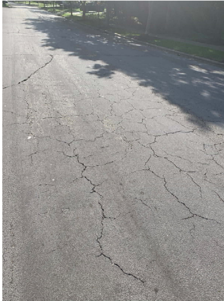
Pavement deterioration (map cracking, longitudinal & transverse cracking)
