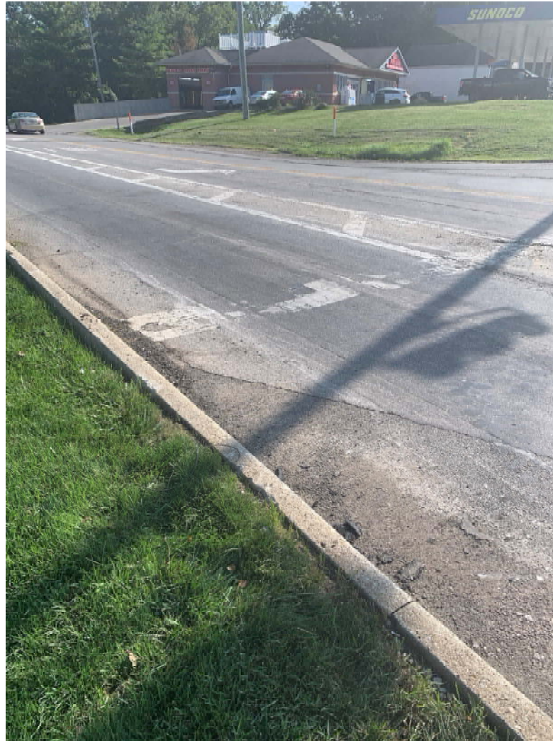
Pavement deterioration (rutting, pavement shoving)
