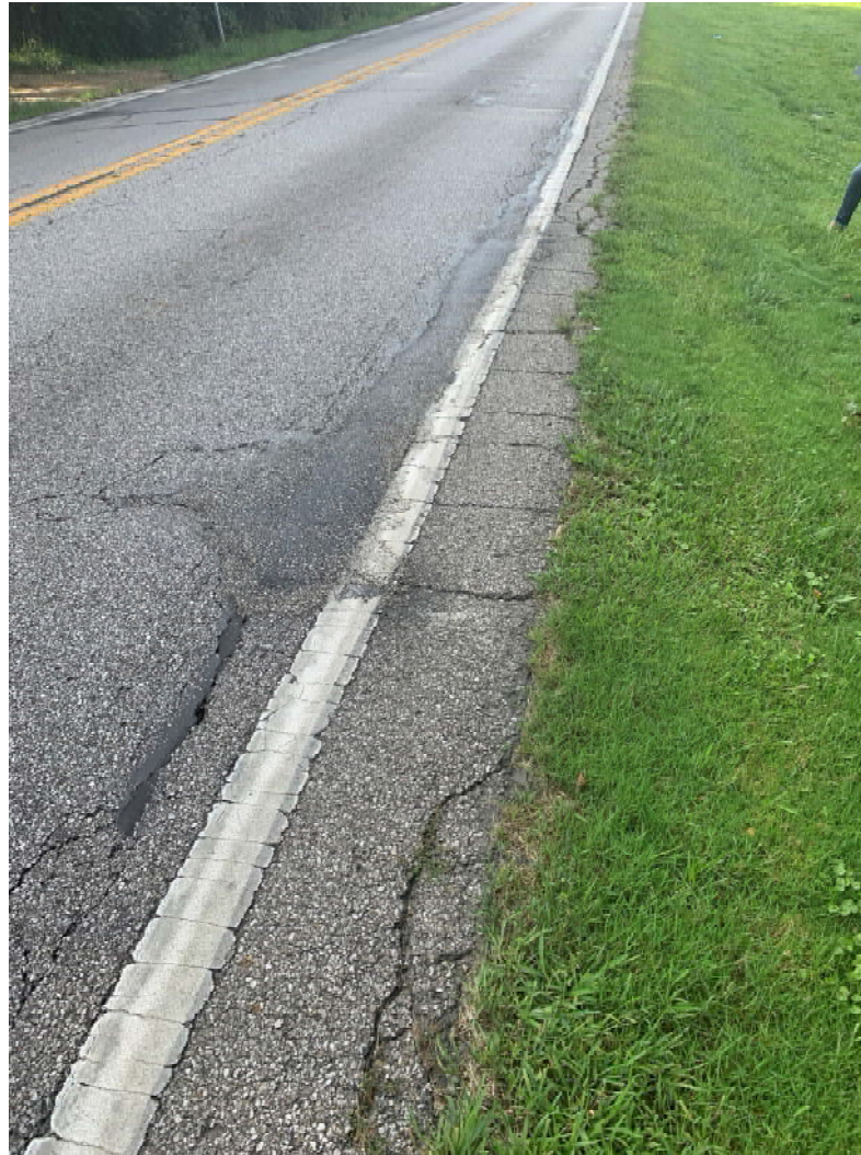
Pavement deterioration (edge cracking, map cracking, patching, rutting)
