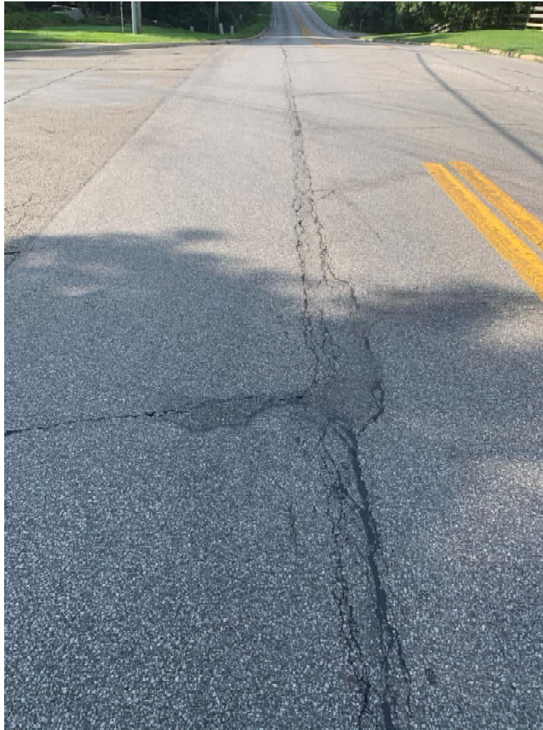
Pavement deterioration (longitudinal & transverse cracking, patching, map cracking)
