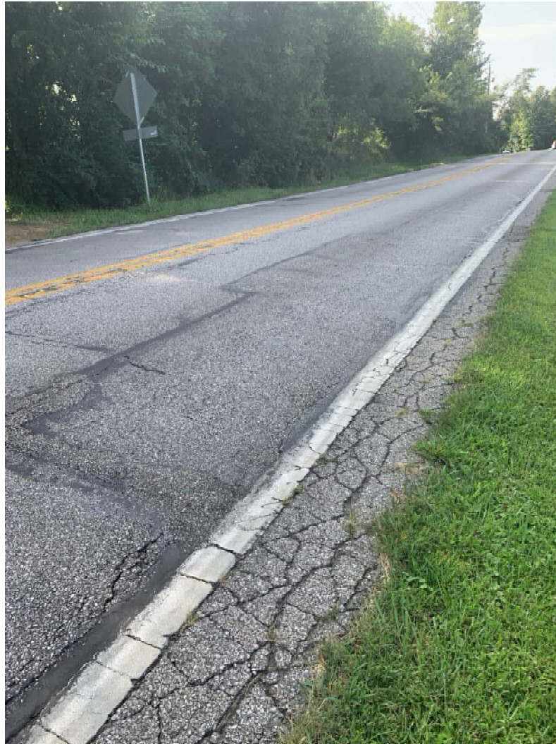
Pavement deterioration (transverse & longitudinal cracking, map cracking, edge cracking, patching)
