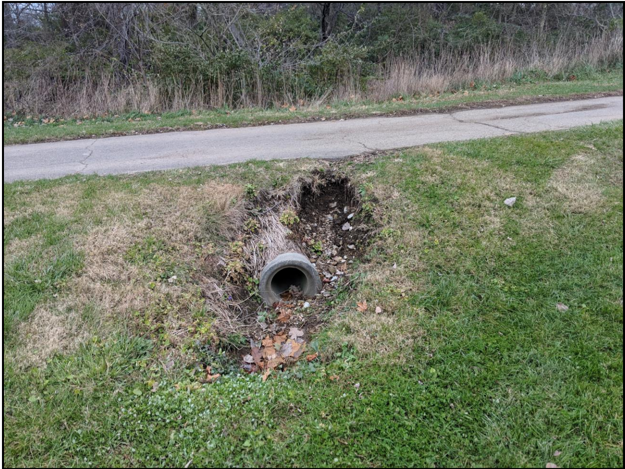
Image 3: Existing erosion at 12-inch diameter culvert inlet.
