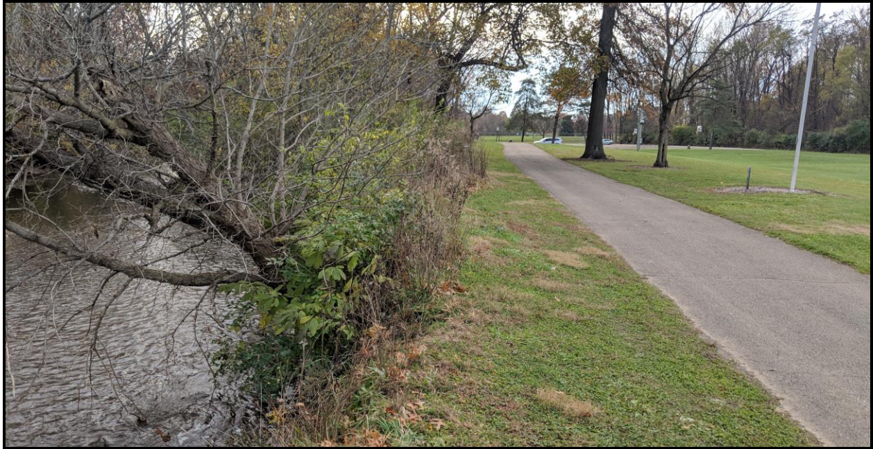
Image 5: Existing streambank erosion near ballfields.
