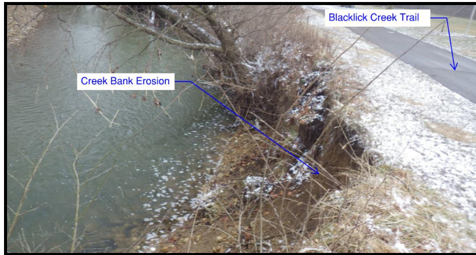
Figure 1: Stream Bank Erosion in Close Proximity to Blacklick Creek Trail
