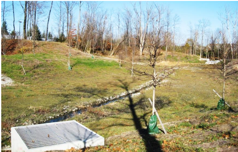
Basin to reduce peak storm flows
