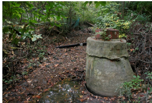
Infrastructure in channel cut by stormwater
