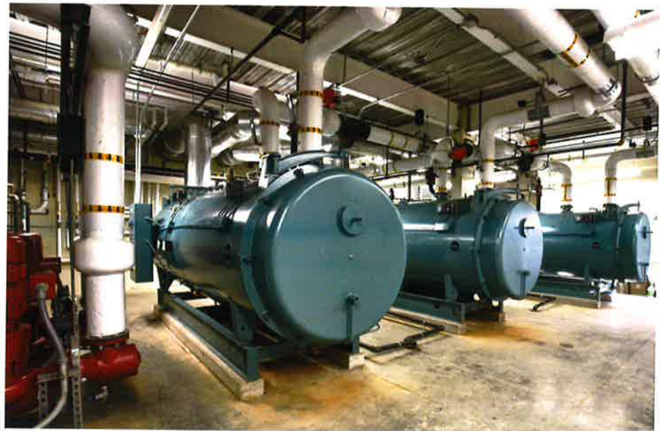
ITHACA COLLEGE MECHANICAL ROOM // KORDA
