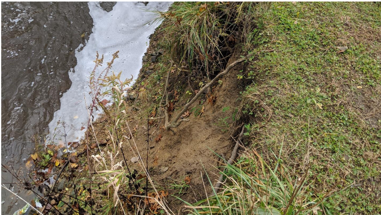
Photo 4: View of eroding bank along Blacklick Creek in Location 2 (EMH&T, 11/13/18)
