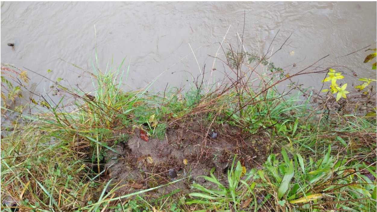
Photo 2: View of collapsing bank along Blacklick Creek in Location 1 (EMH&T, 11/13/18)
