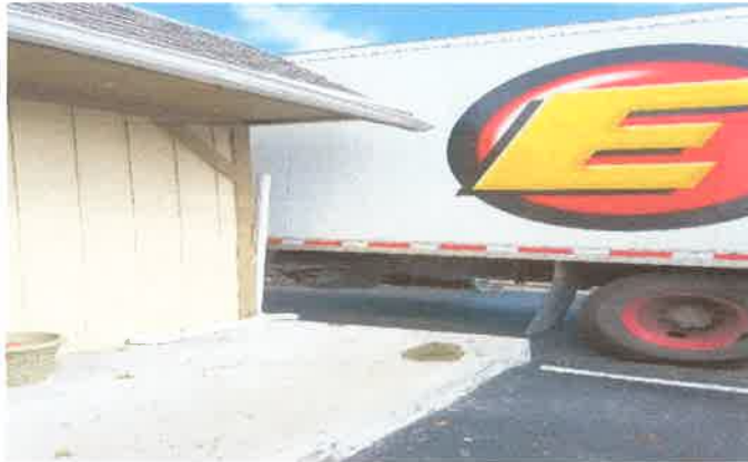
semi truck hit building March 2017
