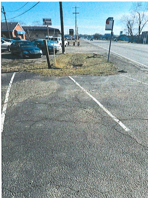
PHOTOS SHOWING CONDITION OF PARKING LOT AND DRAINAGE CATCH BASINS INLETS ON BOTH SIDES OF PARKING LOT ENTERANCE...
