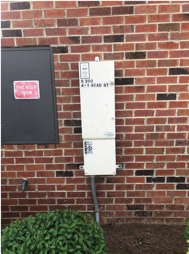
Figure 10. Splitters in Outdoor Cabinets
